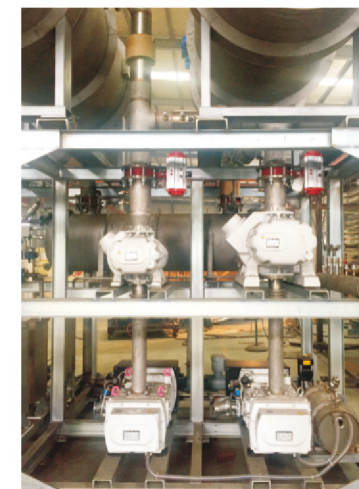
两套维持真空系统 Two sets vacuum maintaining systems
